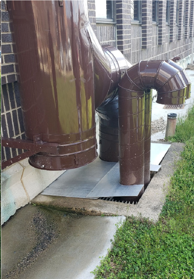
Intake/Exhaust Vents at Area South Facade
