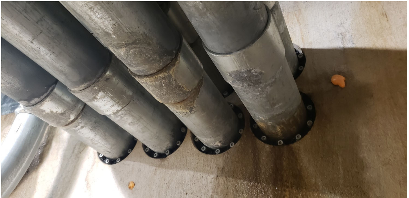
Electrical Feeder Conduit Penetrations at South Facade - Interior
