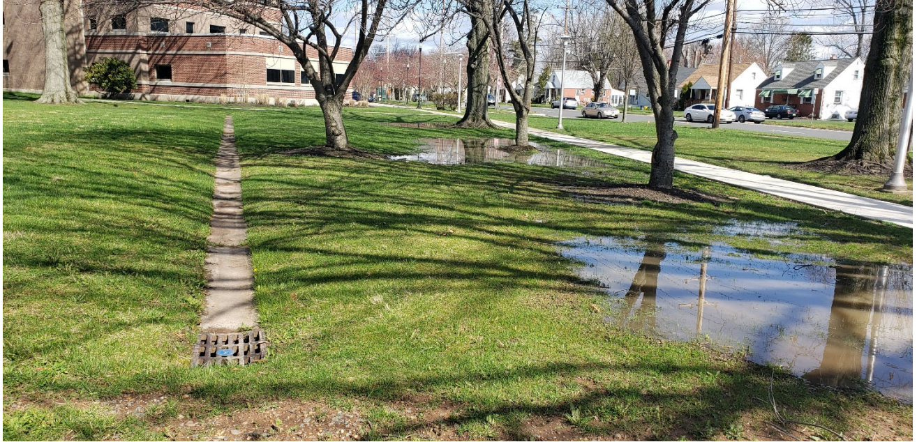
Standing Water and Improper Grading at North Side of F&A Building
