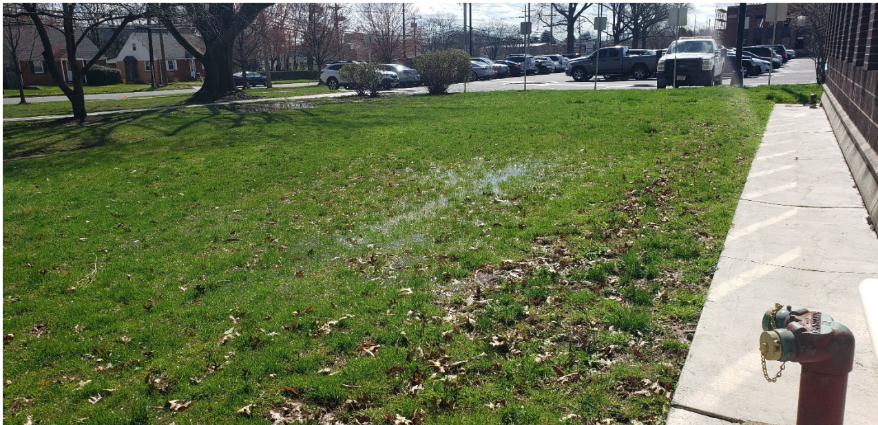
Standing Water and Improper Grading at North Side of F&A Building
