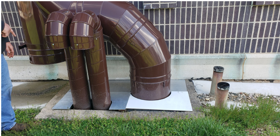
Intake and Exhaust Air Ducts at Areaway at West End of South Wall
