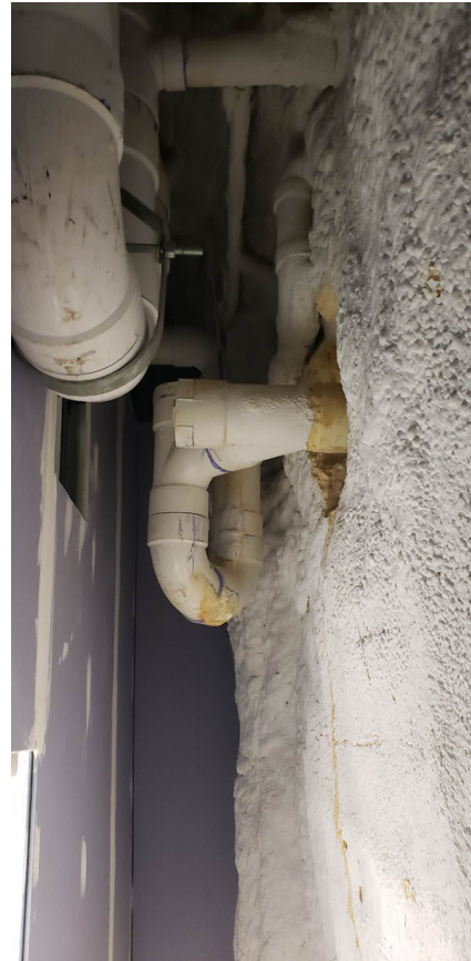
Sanitary Piping Penetrants at North Wall
