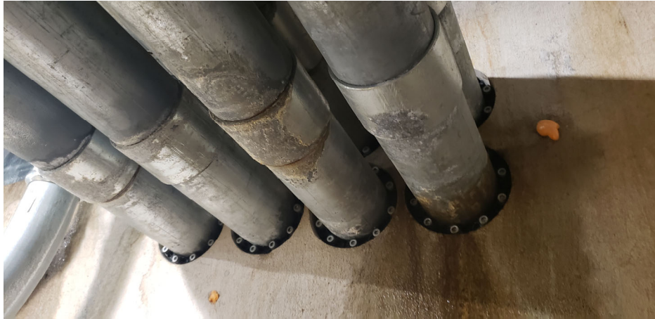
Eight 4" Diameter Electrical Feeder Conduits Penetrating the Foundation Wall at the Southwest
