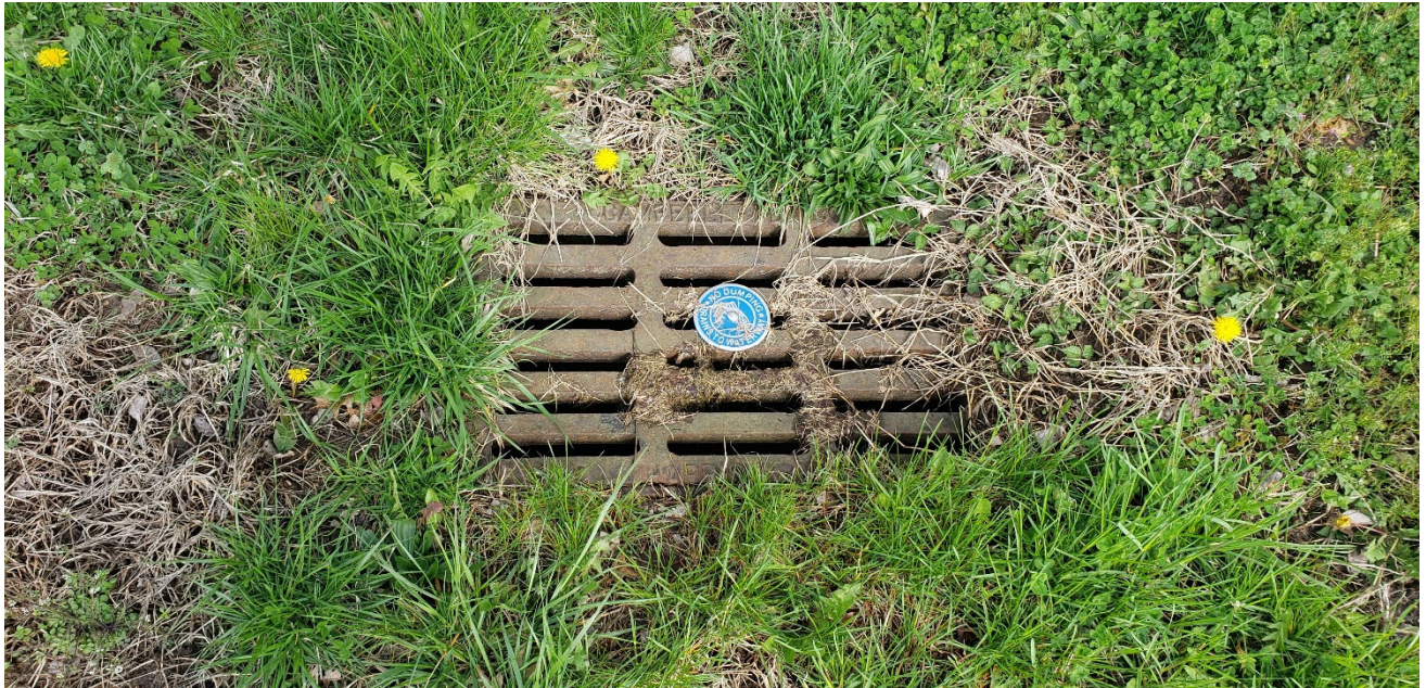
Typical Yard Drain / Catch Basin
