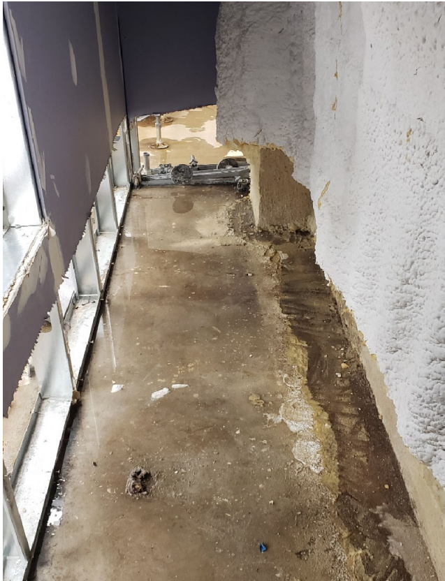
Moisture Along Base of North Wall
